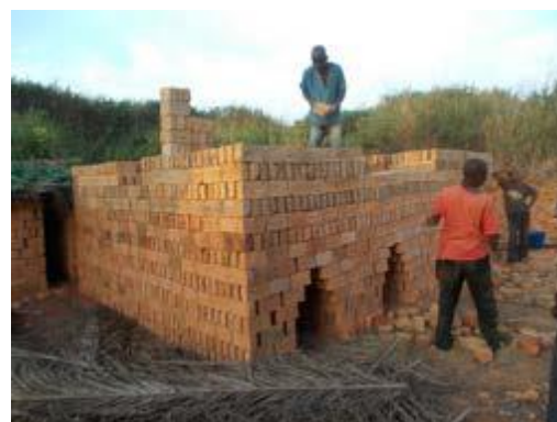
The kiln built by Butoke to make bricks for the school building.
